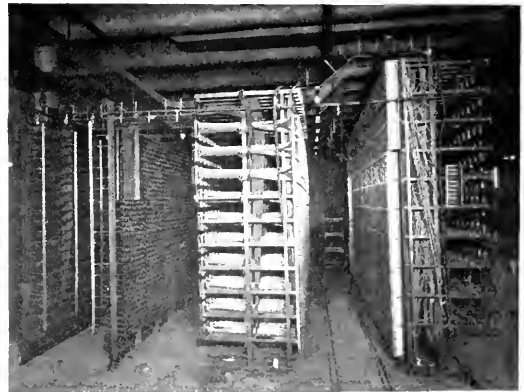
FIG. 3.—MAIN, INTERMEDIATE AND RELAY RACKS, MAIN EXCHANGE.
